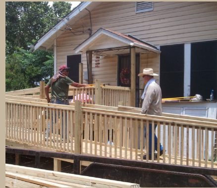
Eight St. Philip's College employees completed a special access ramp as a goodwill project in the city.
